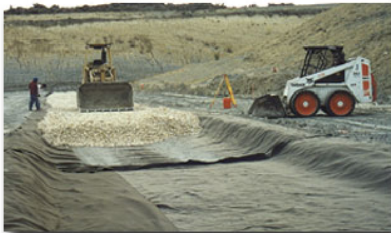
After excavating a landfill site, TDS digs a leachate collection trench and lays down rock and gravel. Liquid will drain into the trench and flow to a low point, where it is pumped out for treatment and disposal. / Photo by Texas Disposal Systems
