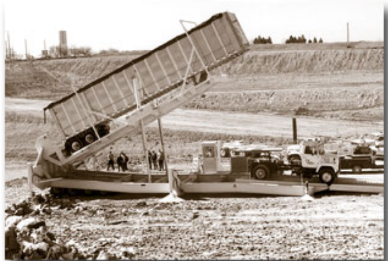
The TDS landfill receives about 2,000 tons of solid waste each day, mostly from Austin and San Antonio. The hydraulic lifts on trailer tippers raise semitrailers high in the air to empty the contents. These long trailers transport a volume equal to three or four garbage trucks. / Photo by Texas Disposal Systems
